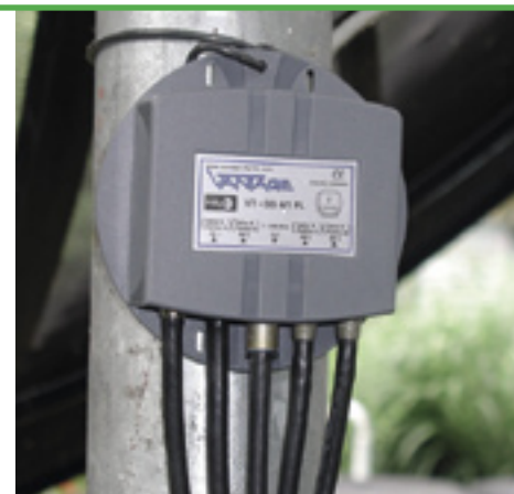
DS 4/1 PL switch connected to the same 10-foot dish plus two additional antennas
